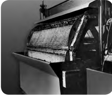
Traveling water screen.
